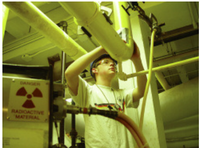
Brian Neemann setting up isotope radiography equipment to inspect a piping weld on the college's heating boiler gas manifold system.
